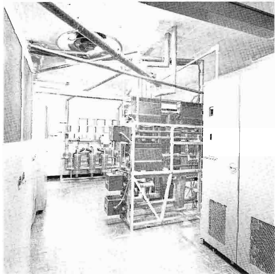
New TV-12 transmitting system includes OPTO-Switcher for optimum VSWR. Entire system was optimized on site before going on-air.
